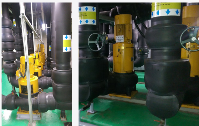
Pump body and piping with black color insulation material are used as chilled water pumps, those without the black color insulation are condenser water pumps.
