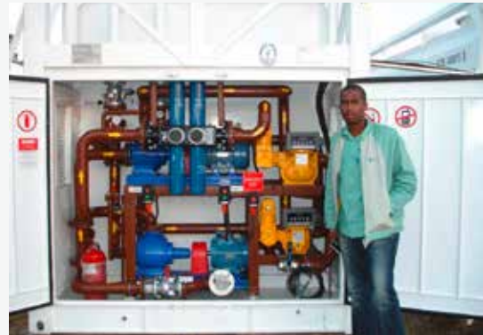
Company Self Bundled Tank Trailers in front of the fuel unit with the DESMI Modular S pump installed
