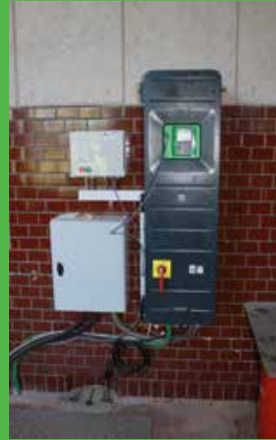
Schneider frequency converter installed at Lumby pumping station.
