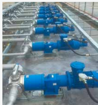
The eight DESMI ROTAN® pumps at the production plant in Jinlong Industrial Zone (Guangzhou, P.R. China) which is the most famous area for coatings.
