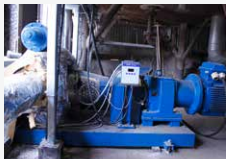
ROTAN® HD152EDDKLT-1U22S in NCC's plant in Roust
