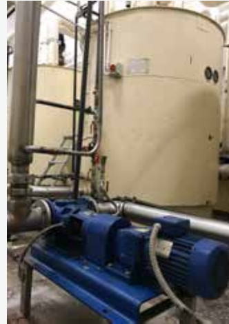
One of the DESMI ROTAN® HD (HD66ECHD-1M22B) internal gear pumps installed in the Carletti factory in Pruszków near Warsaw, Poland.
